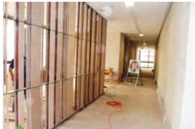
The Phahon Yothin Main Branch, established more than 25 years ago, is under renovation for energy saving
